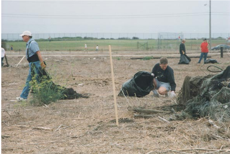
In anticipation of City approval, volunteers remove debris from the White Point property. Over 45 tons (yes, tons) were removed after the first cleanup day.
